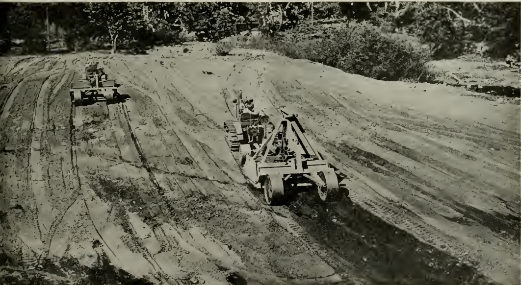
Seven-yard scrapers spread fill material on dam. Weight of earth-moving aids compaction of impervious fill, which is completed by twenty units of sheep-foot rollers.
